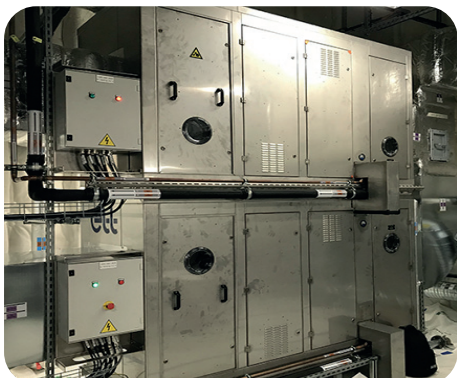
Pressurisation Air Handling Unit (AHU)
