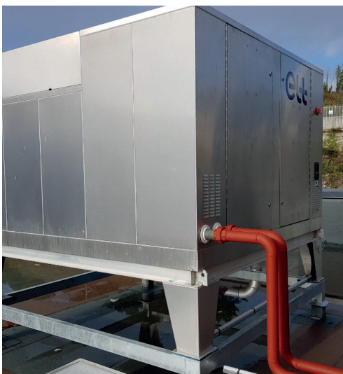
Chilled Water Unit (CWU)
