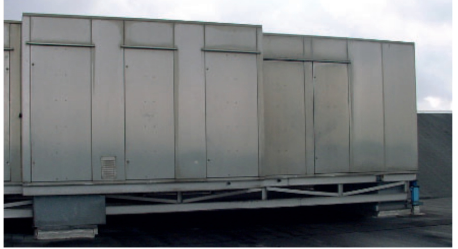
CTA 35 (Air Handling Unit) – Hall Ventilation
