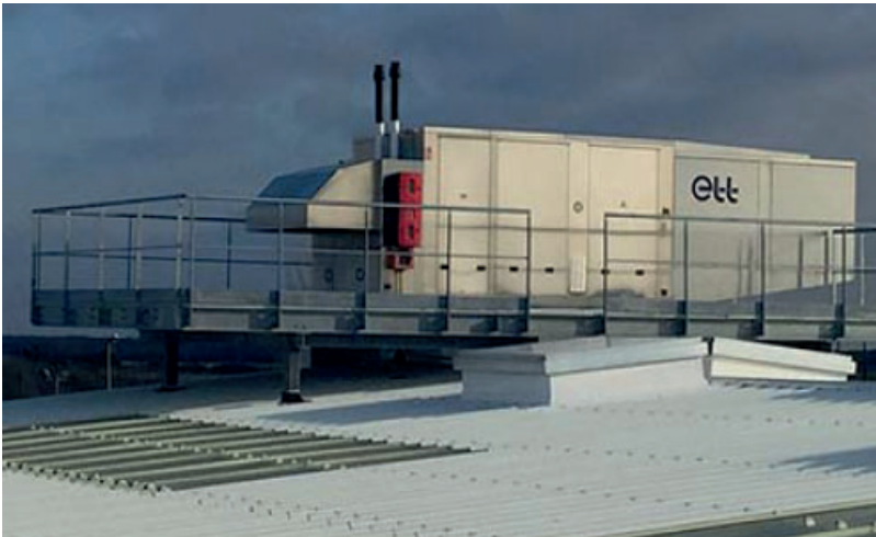
CTA CC+ (Air Handling Unit) for ventilation and heating - Production hall
