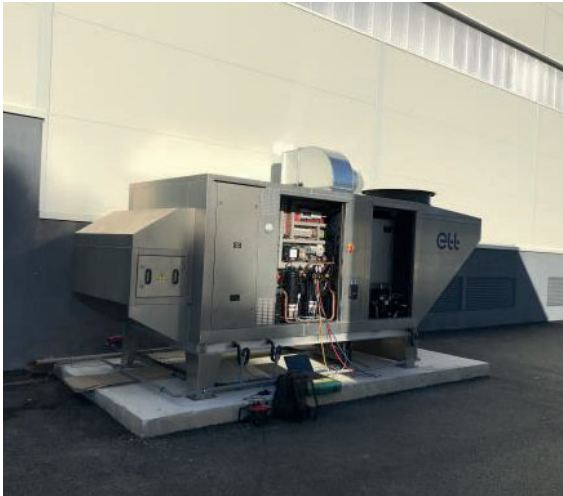
Air-to-air" heat pump for paint shop
